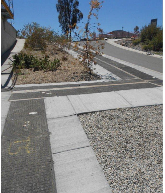
After: Mt. Stromlo Water Treatment works trench runs, repaired with our products.
