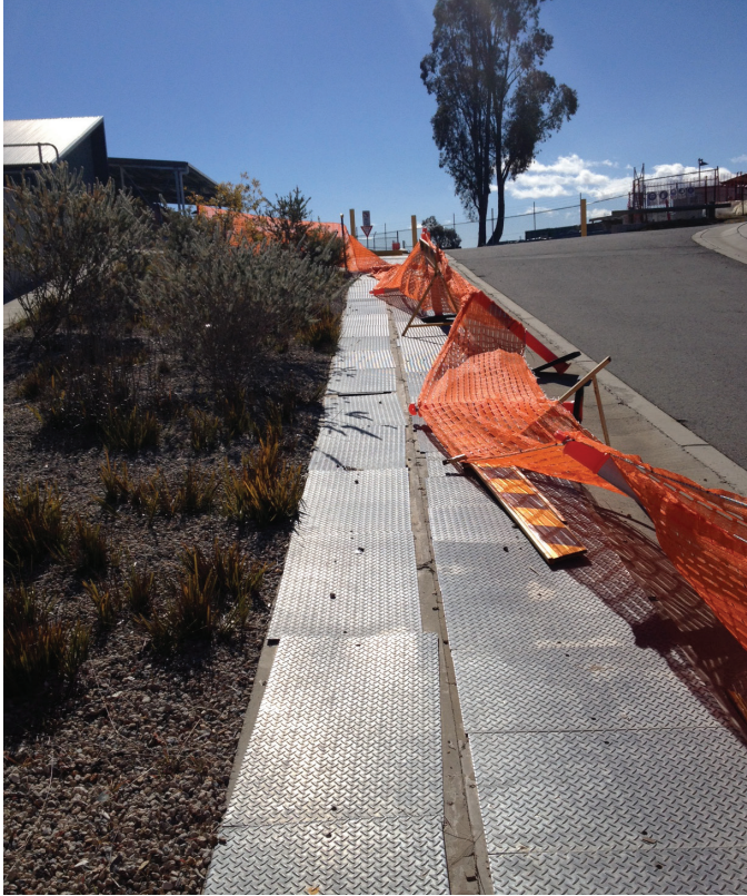
Before: Damaged Mt. Stromlo Water Treatment works trench runs.
